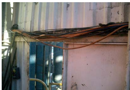
Photo 7 – Poor Dressing of Cables
