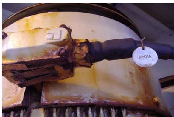
Photo 3 – Corroded Junction Box on Pump Motor
