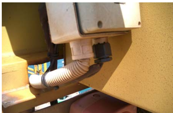
Photo 1 – Damaged Conduit and Exposed Wiring
