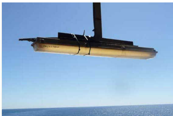
Photo 2 – Poorly Maintained Light Fitting in Process Area
