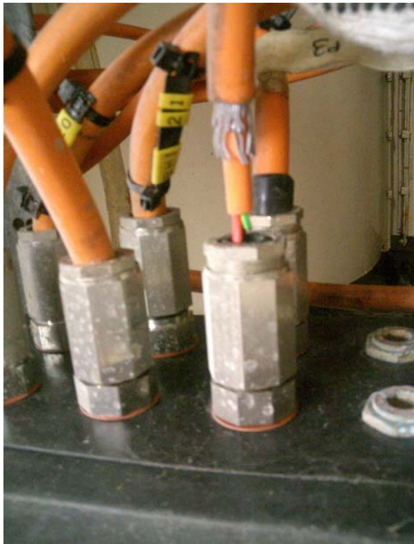
Photo 5 – Exposed Wiring (pulled out of gland)
