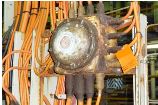
Photo 6 – Corroded Junction Box
