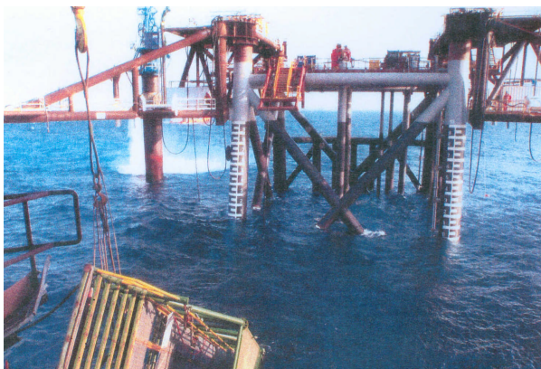
The gangway collapsed into the sea
